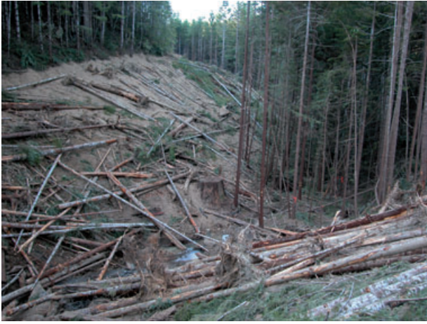
Figure 4. Example of recent road decommissioning. The road prism is extensively reshaped, and some second-growth forest adjacent to the road alignment is cut down to facilitate outsloping. The stream channel crossing is excavated more extensively. The cut trees are left on the reshaped road alignment as mulch.
